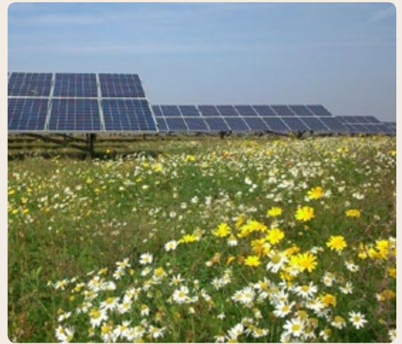
Saxley solar farm, Hampshire
