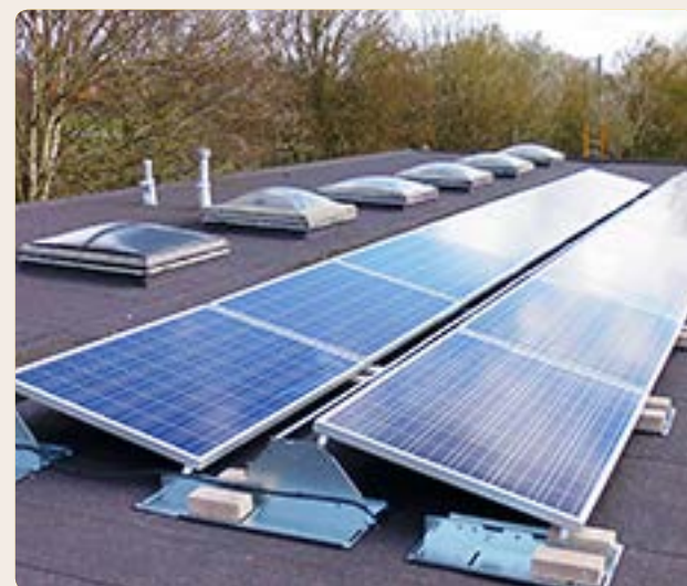
Solar panels on a cricket pavilion in Eynsham
